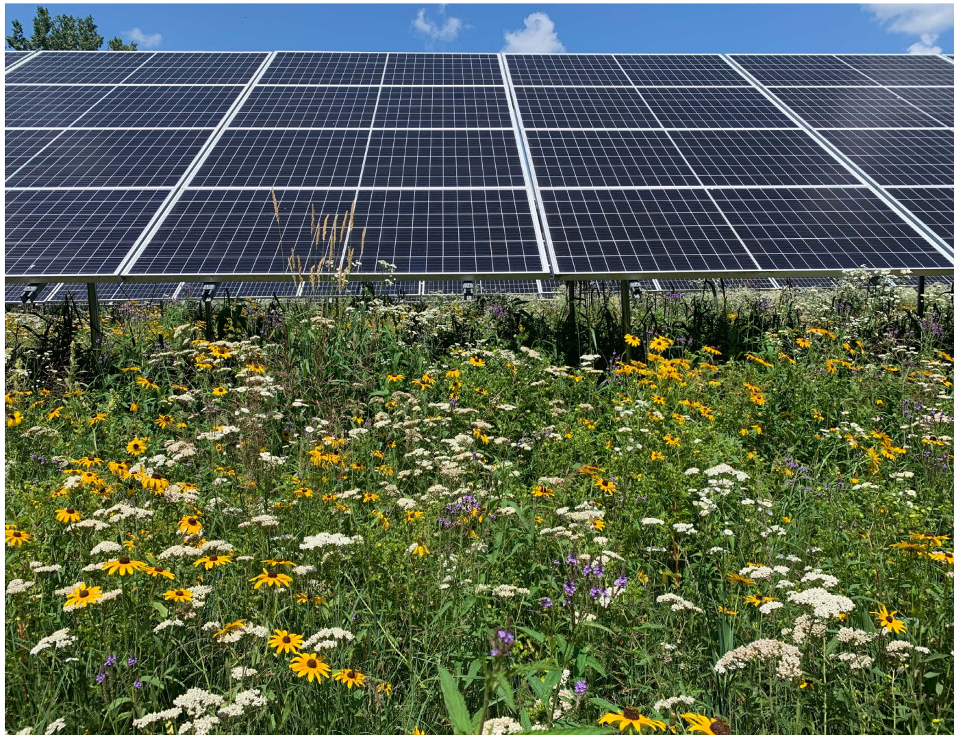
On-site solar and pollinator garden at Melville, New York site.
