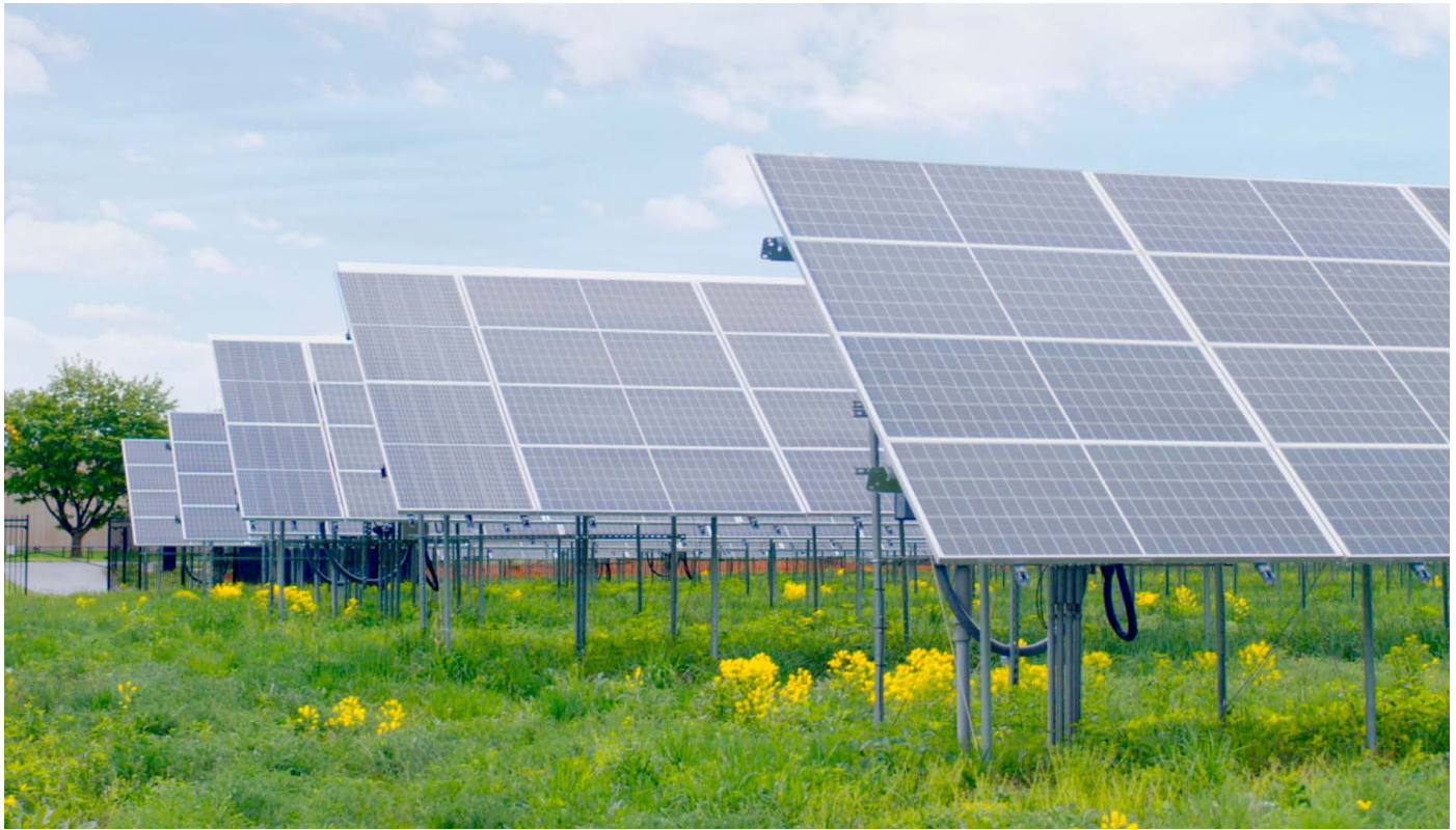
Solar panels at Aveda's Blaine campus in Minnesota, United States.
