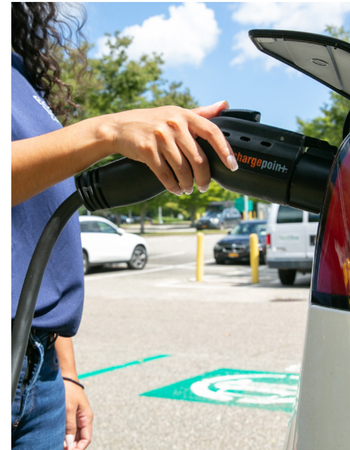
Electric vehicle charging station at ELC's Melville, NY site.
